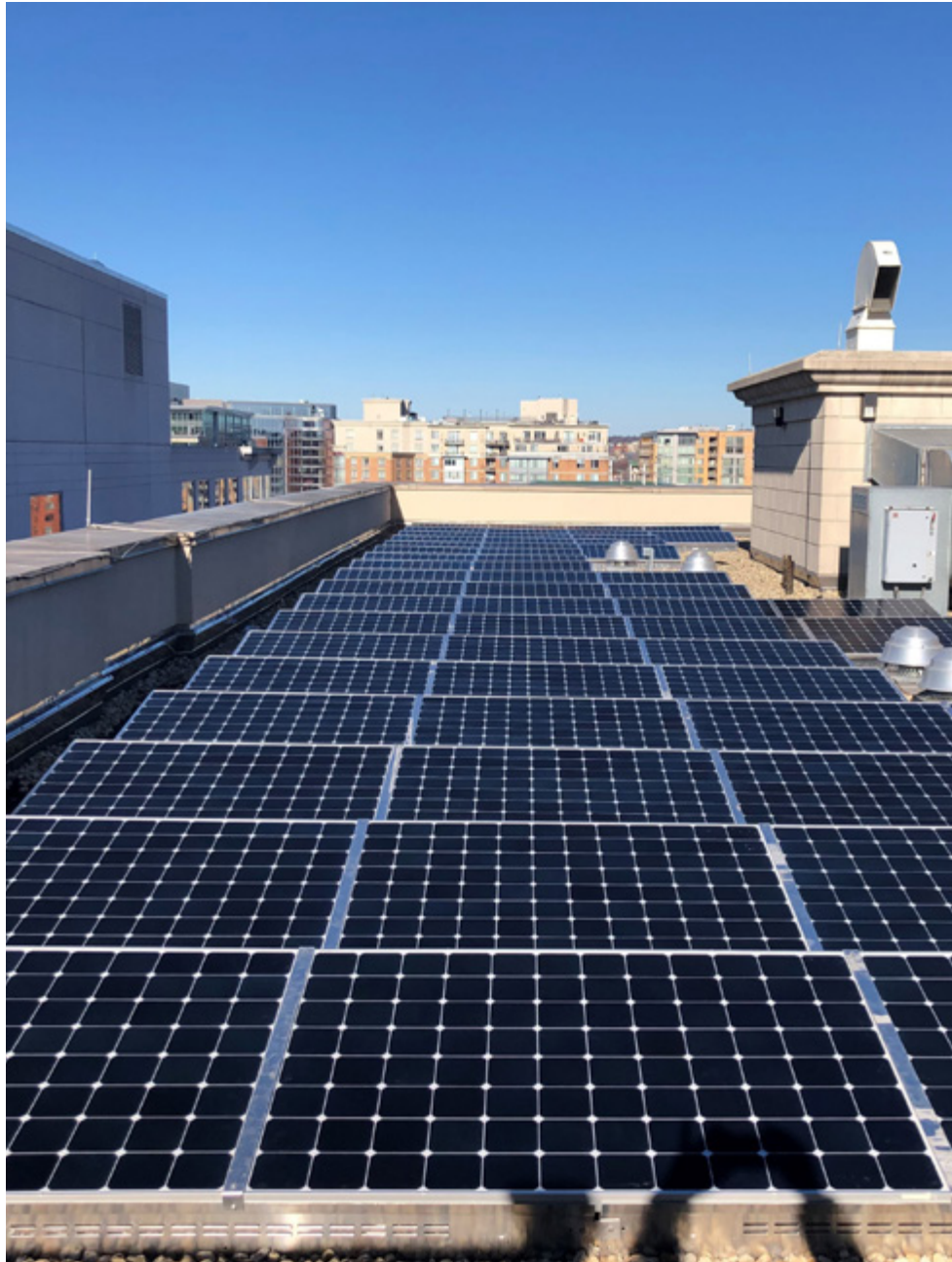
AvalonBay Communities, Inc., Gallery Place Solar Panels, Washington, DC
