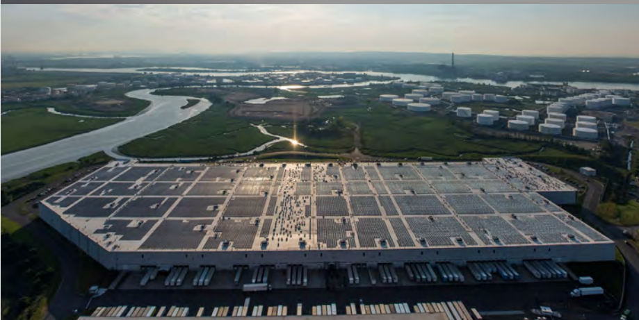
Solar installation on the rooftop of Prologis Park iPort 2, Carteret, NJ, provides 9,000 MWh annually
