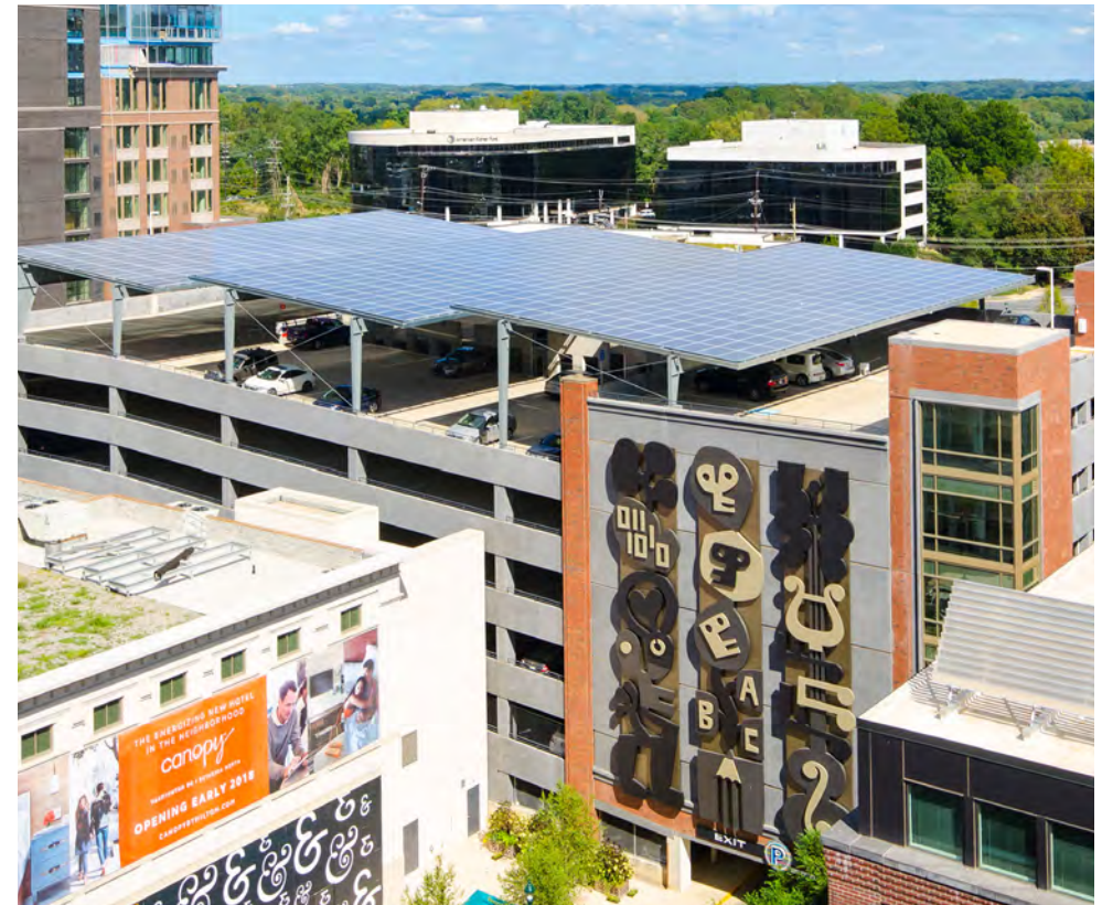
Federal Realty Investment Trust, solar panels at Pike & Rose, Bethesda, MD
