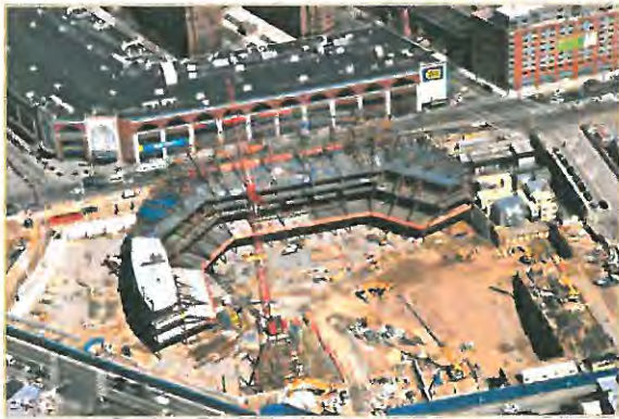
Barclays Center Arena, the cornerstone of our Brooklyn Atlantic Yards project and the future home of the NBA's Nets, is under construction and expected to open in late 2012.
